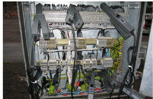
Figure 3 Control cabinet with current clamps
